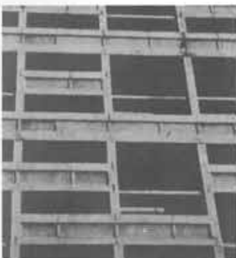
Hierarchy of curtain wall types: Mies van der Rohe, Lake Shore Apartments; Harrison and Abramovitz, Republic Bank, Texas; SOM, Lever Brothers House, New York; Le Corbusier, Unité d'Habitation, Marseille.
