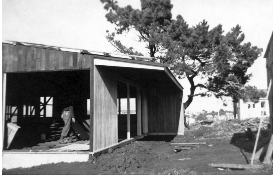
Fig. 1: The First House under construction in 1950. Source: Architecture Archive, The University of Auckland.
