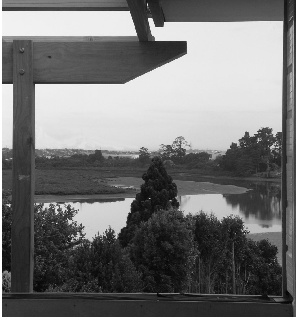
An example of buildings being droll: the Adams Cheng Residence under construction, Avondale, Auckland. Photo: Cheng.
